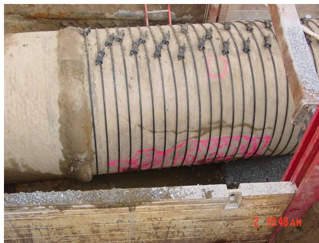
Figure 6: GLSD Pipe Section 22
