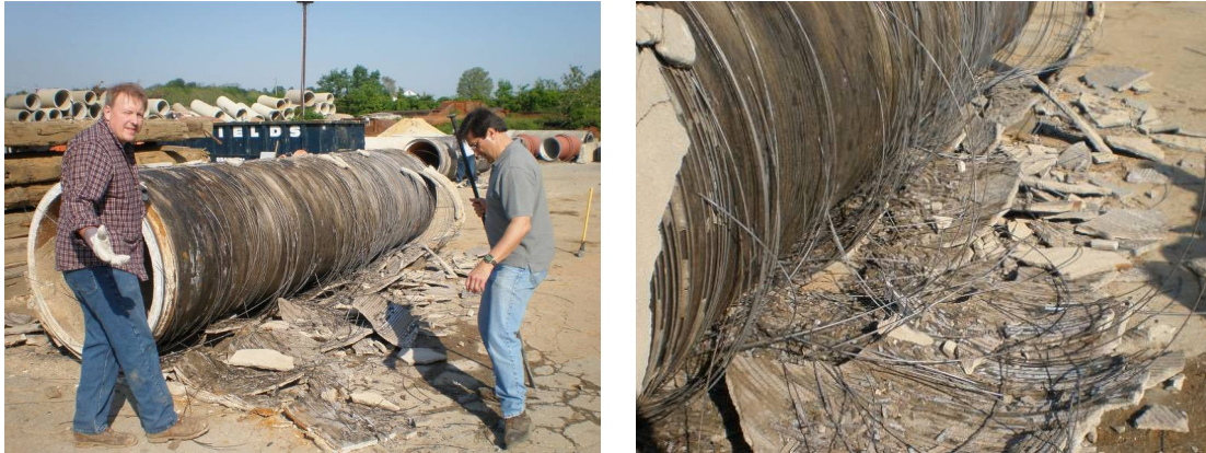
Figure 5: Ridge road main in Howard County
