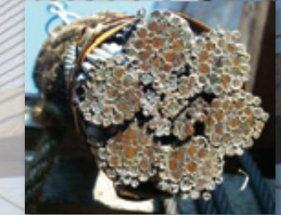
Corrosion and deterioration generally originates on the inside of the wire rope.
