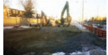
Crews working on the broken water main in Woodroffe Avenue in January
